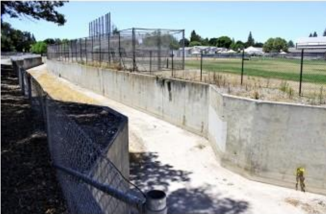
Figure 8. Permanente Creek Diversion Channel constriction. View is upstream and generally to the west. Blach School is in the background. (Water District, n.d.)
