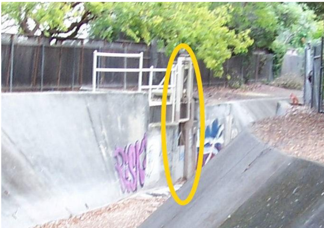
Figure 7. Permanente Creek Diversion Channel floodgate/valve. View is downstream and generally to the northeast. The yellow ellipse contains the floodgate. (Grand Jury, October 28, 2015)
