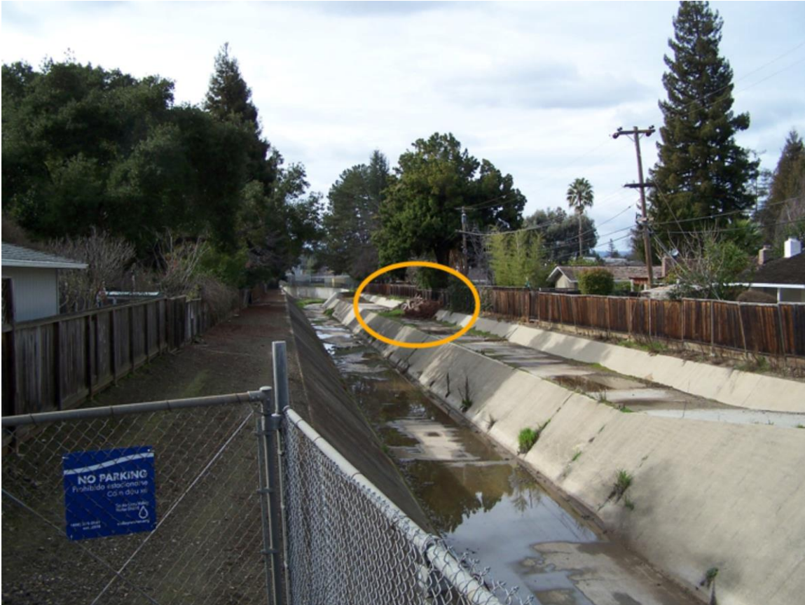
Figure 9. Debris on the shoulder of the Diversion Channel upstream of Grant Road, Los Altos, facing west (Grand Jury March 1, 2016)
