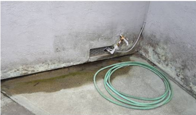
Figure 2: Foundation—Leak and Black Substance
